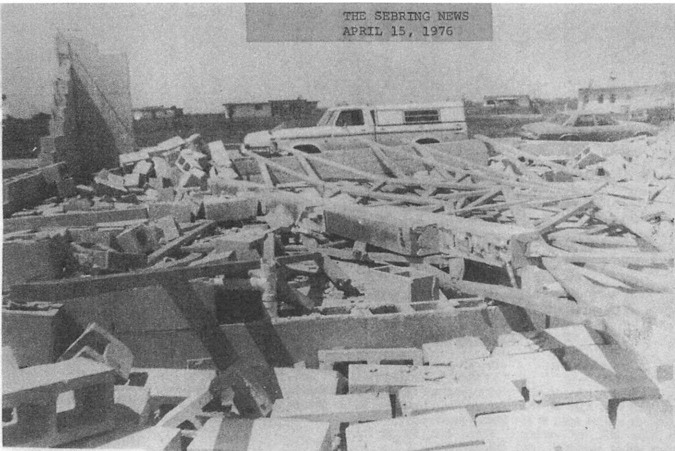
The walls and wooden braces of this house under construction at Spring Lake Village 2 were leveled by the force of the tornado. When the storm had departed, only one wall was left relatively unscathed. Newsphoto by Wadlow.
